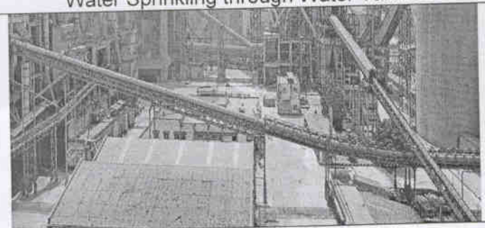
Closed Conveyor Belts
